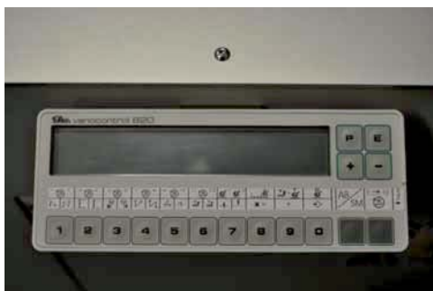
Common control box and panel for all units
