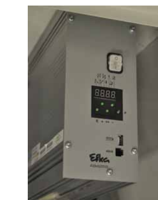
Common control box for all units
